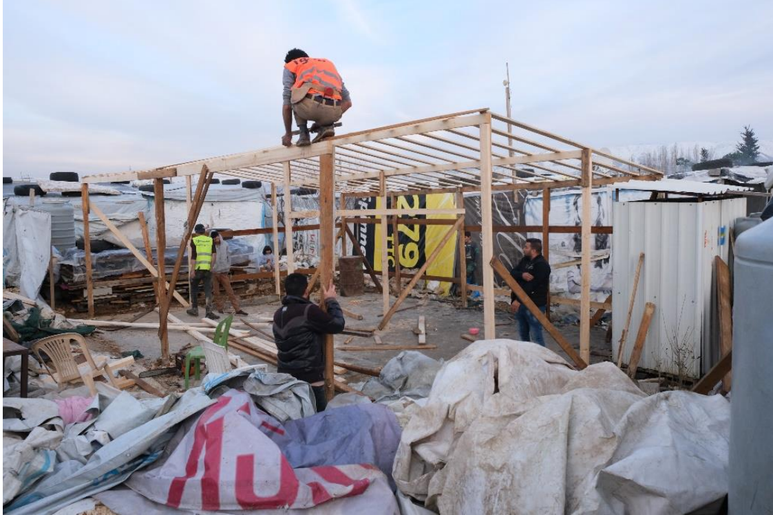
Pic9: Saadnayel- SAWA's team with volunteers from the community during rebuilding damaged tents by using woods, shaders and many other materials provided in this project.
